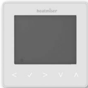
Thermostat completely OFF
